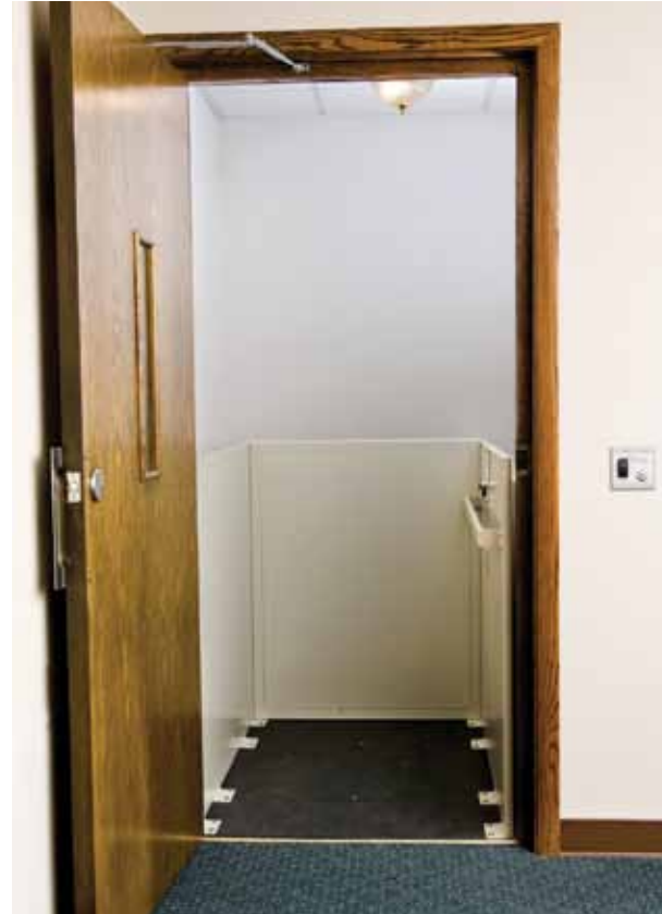
BC Model with runway enclosure built by others and non-fired rated wood door
